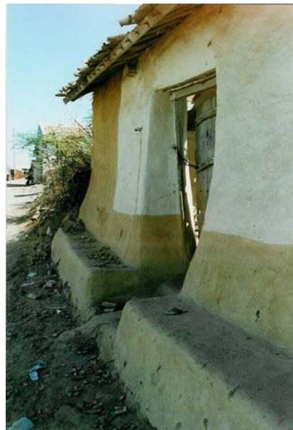
Building Construction. Fig. 16 Mud wall in a tapered form to withstand horizontal earthquake forces (Gujarat, India) (photo by the author).
